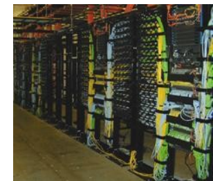
Today's Networking Equipment.
